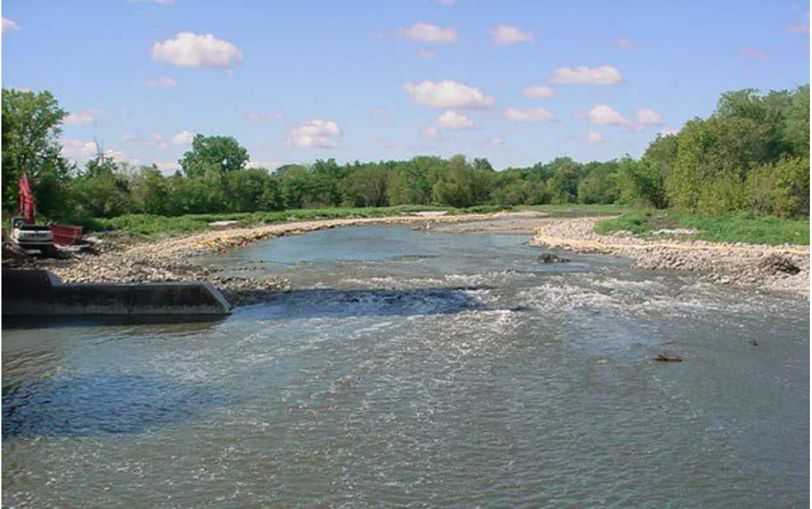
Figure 8: Removal of the Hofmann Dam with 30 foot long section remaining on right bank, looking upstream (IDNR)
