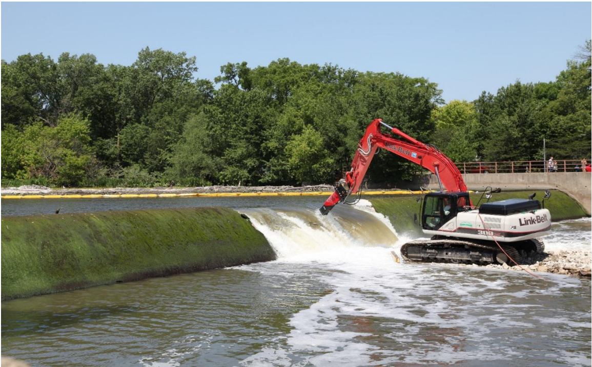
Figure 7: Notching of the Hofmann Dam, June 2012 (IDNR)
