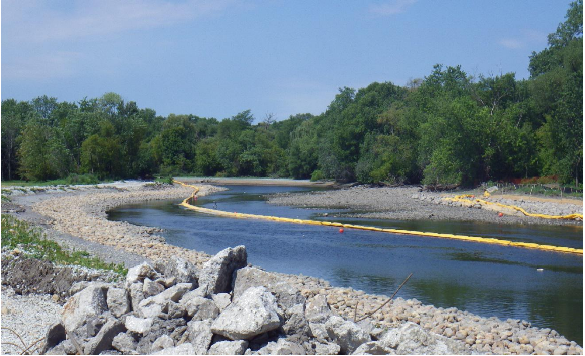
Figure 10: Riprap and silt turbidity curtain installed in the former Hofmann Dam impoundment (IDNR)
